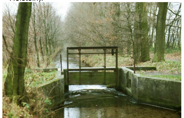
FIGURE 3.6: No reference site: the migration of fish and invertebrates is obstructed by a weir (Dellbach, Lower Rhine area).
