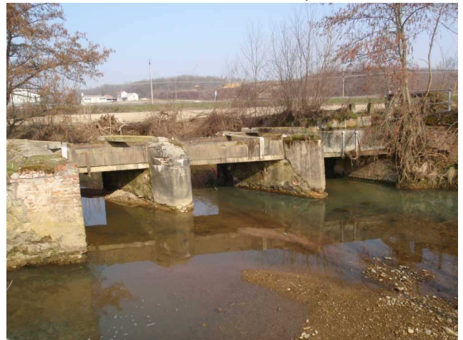
Special features/Neglected bridge - Guarabione Sdop, 10/05/2011.
