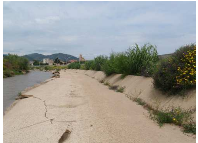
Special features/ Reinforced channel – Foddeddu Valle, 21/05/2011.
